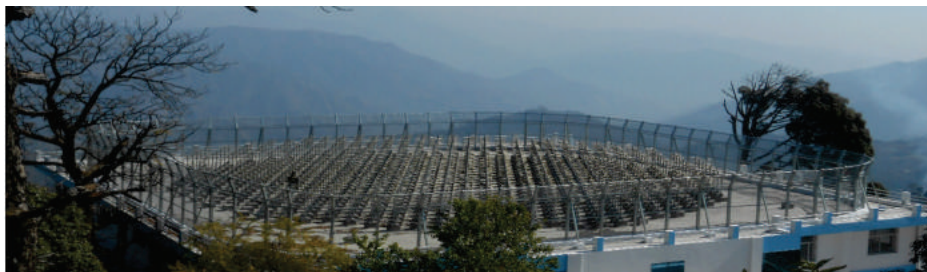
ASTRAD antenna array on the roof-top of the ASTRAD building with recently installed clutter fence along the periphery of the antenna array.
