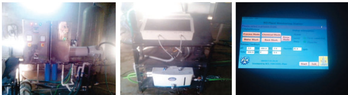
RO plant with controller system
