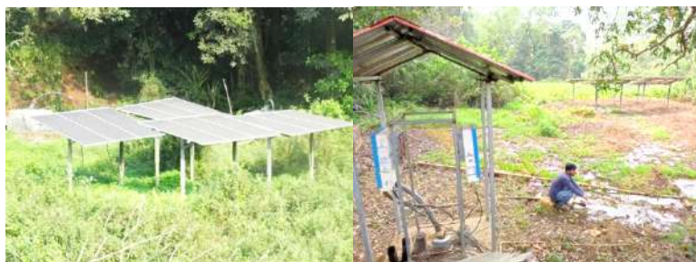
Fig. Solar-powered RBF wells at Cortalim, Chaudder lake Goa
