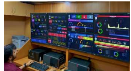
Fig. SoC C3iVazra installed at NHAI
