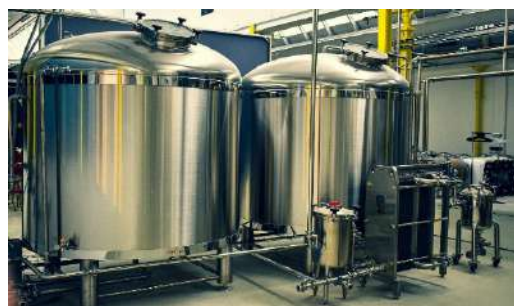
Fig. EffluePure effluent treatment plant
